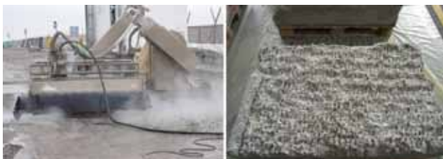
Figure 2. Treatment of top concrete surfaces of blocks A and B with water under high pressure (hydro-demolition)
