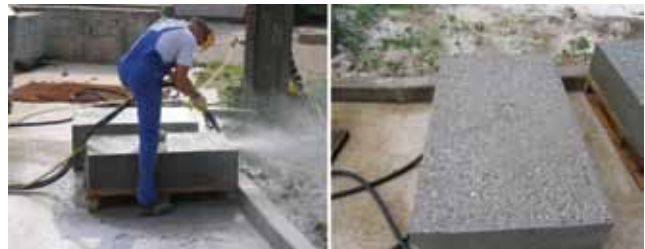
Figure 4. Top concrete surfaces of blocks A and B subjected to water jet treatment with sand (sandblasting)
