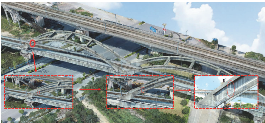
Figure 18. Blooming of the arch surface
