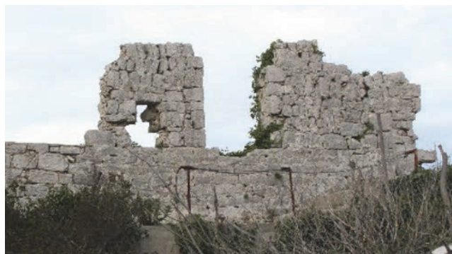
Figure 11. Opening and two merlons of the north-wall crenellation, damaged arrow loop is visible at the left-side merlon
