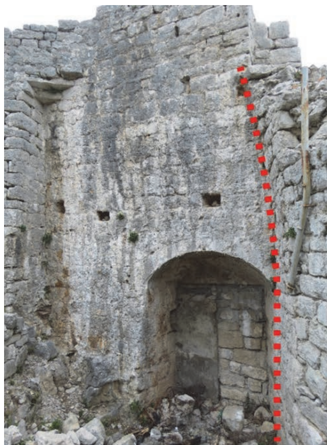
Figure 14. Cantilever part of the defence wall next to donjon and S-E tower
