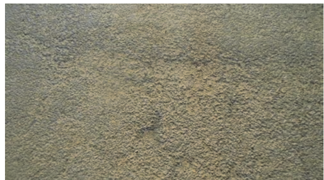
Figure 6. Road surface in October 2015
